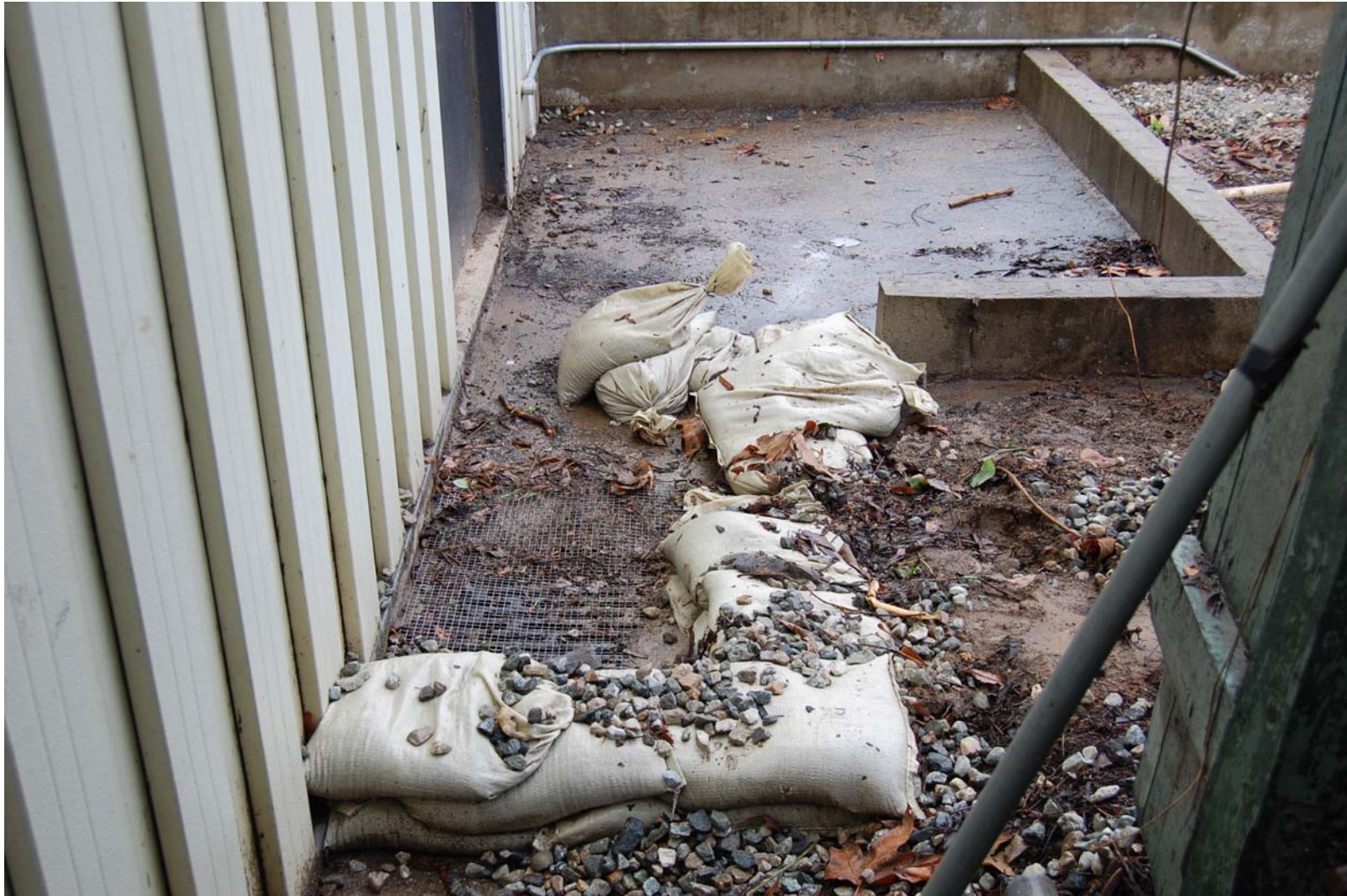
A very helpful man from Physical Plant arrived to unblock the drains whilst we attacked the water inside with his Shop-Vac.
