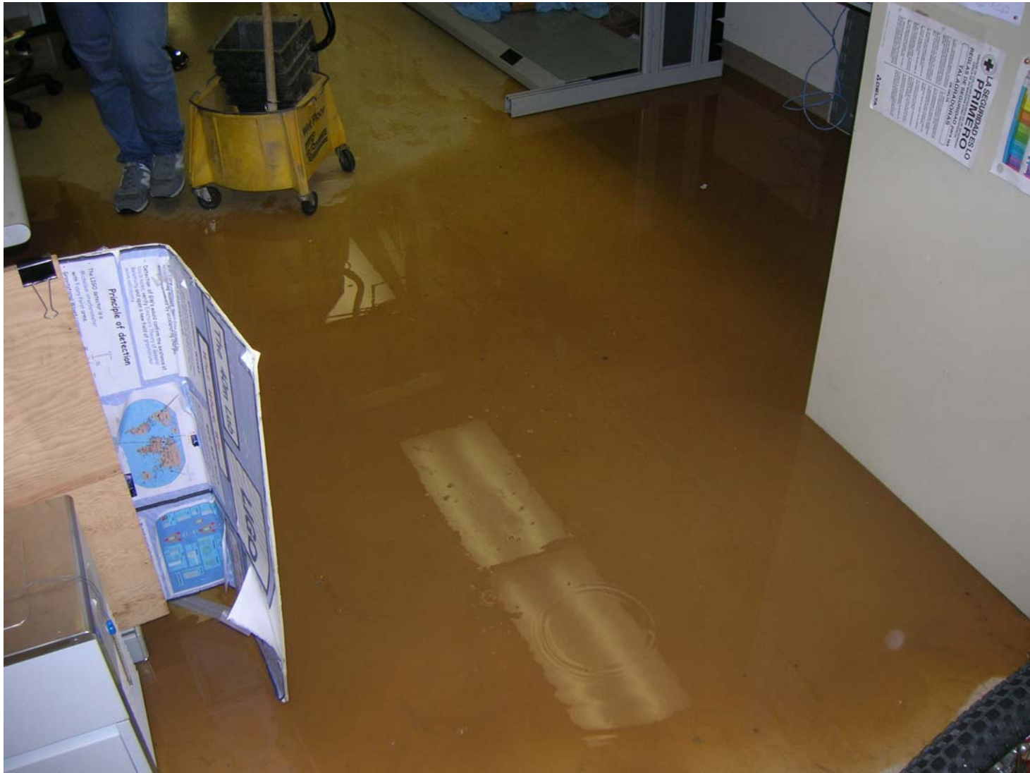
This lead to a little bit of moisture entering the control room...
